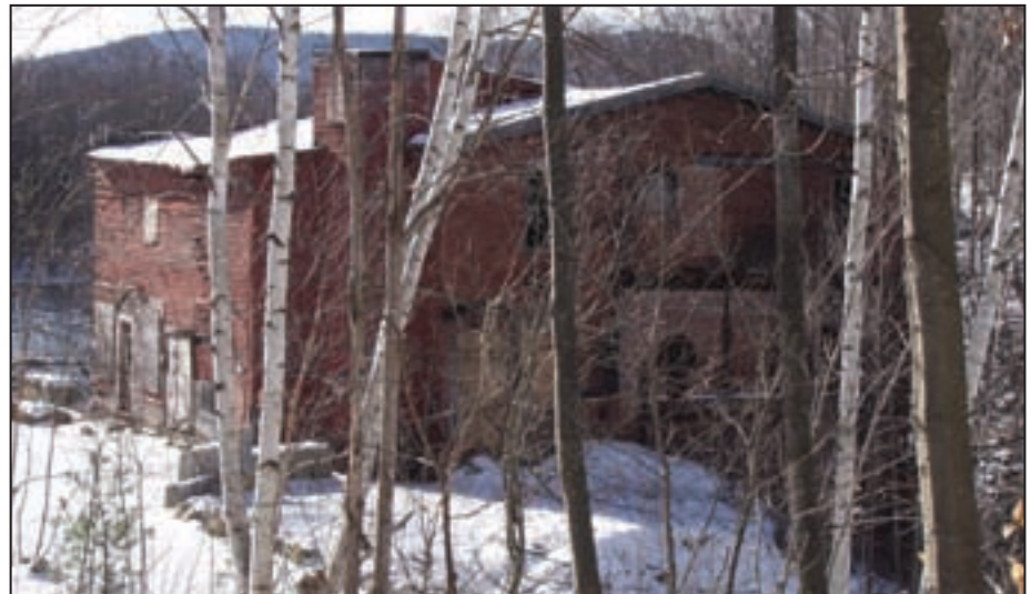
Demolition of the former Woods Woolen Mill was halted because of hazardous materials on site.
