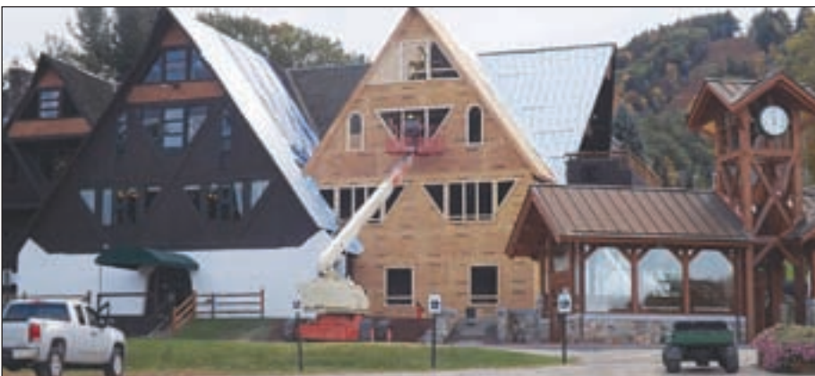
Pats Peak is making renovations in anticipation of the new ski season.
