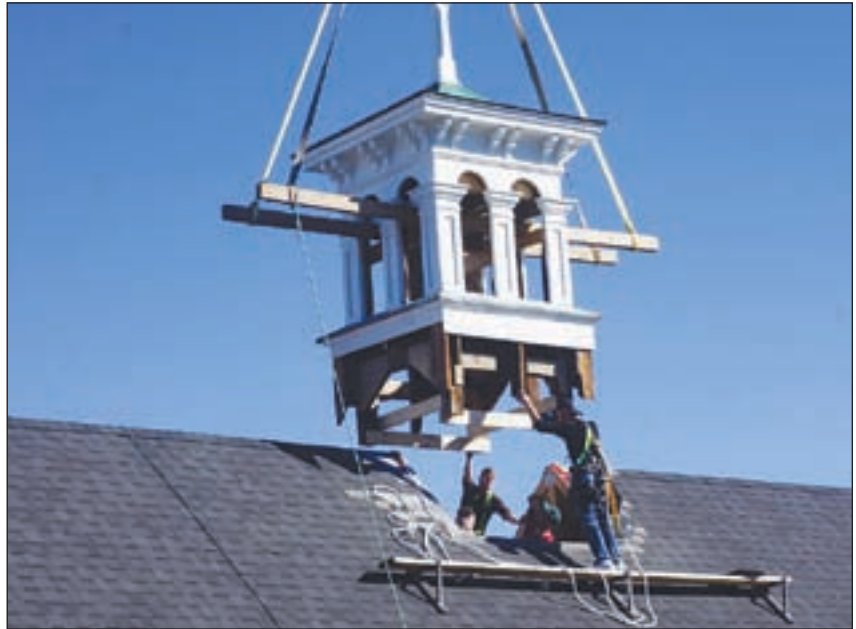
Topping it off. Workmen reinstall the cupola 364 days after it was removed.
