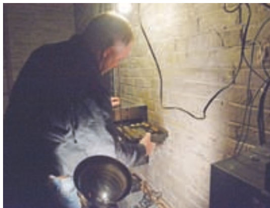
President of the Newport Opera House Association David Hoyt pulls out a circuit board of one of the dimmer boxes to show that it is burnt out and the cause of the electrical problems that have made the house and stage light to go dark. The Newport Opera House Association is looking into estimates to repair, upgrade or replace the lighting system.
