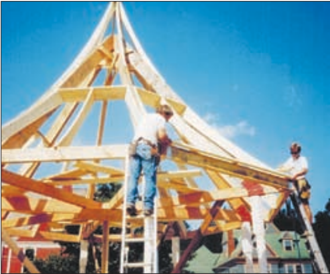
New Boston residents Tony Hall and Tom Condon building the New Boston Gazebo in 1994.
