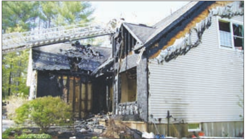
Fire caused substantial damage to this Weare home.
