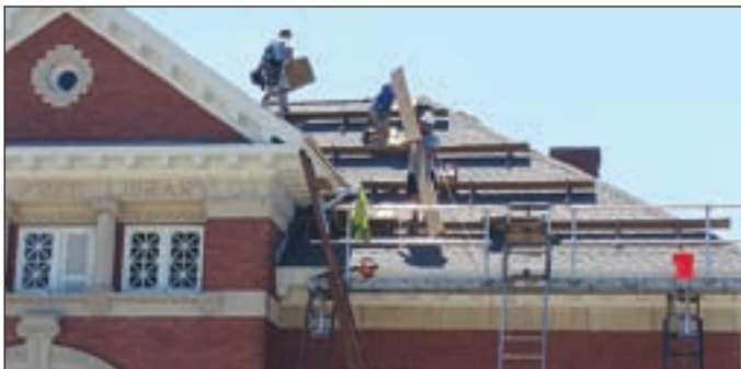
Workmen are busy installing a new roof on Henniker's Tucker Free Library.
