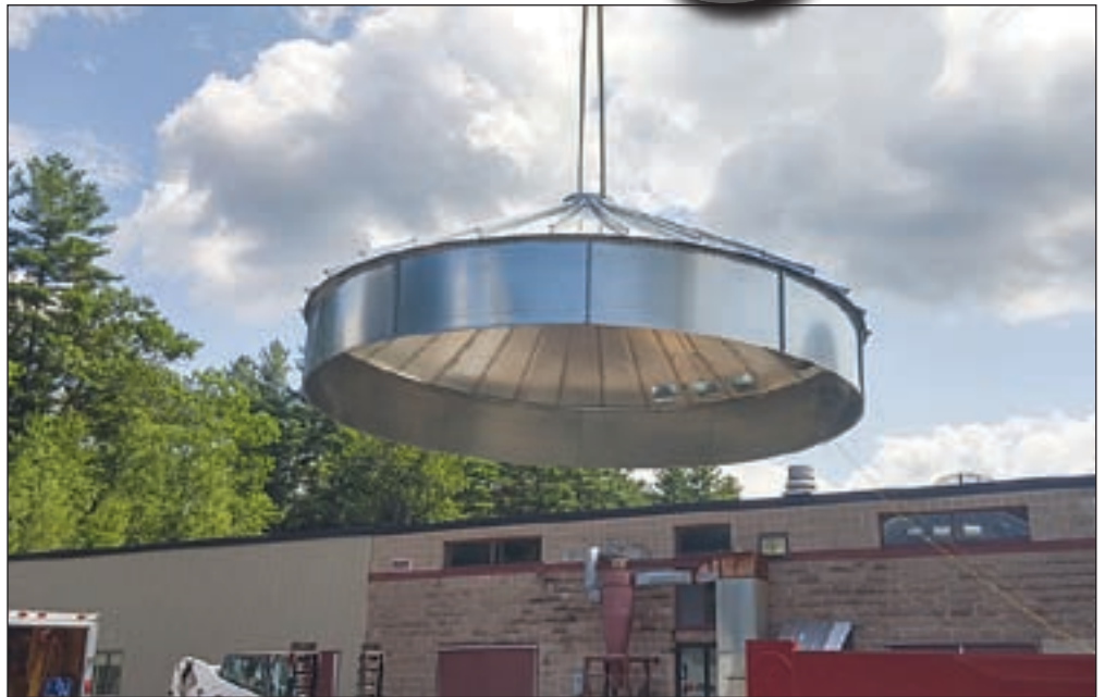
The wood chip silo for the biomass project has been installed. John Astholz photo.
