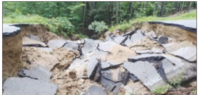
Peterborough's Middle Hancock Road is still closed. Due to extensive damage and availability of resources, repair will not begin until Thursday, August 30th.
