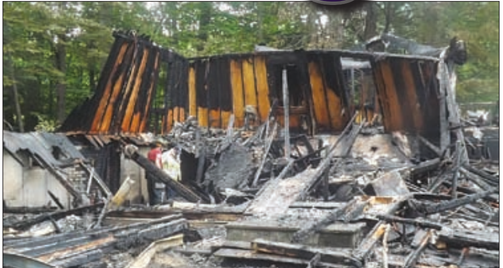
Hillsborough Firefighters could do little to save this home on Deer Lane. By the time they arrived, it was fully involved.
