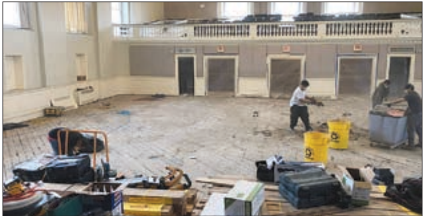
Work has begun on the Upper Hall floor of the Peterborough Town House, rebuilding the wood floor just in time for Veterans Day, and the ongoing celebration of the Centennial of the Town House.
