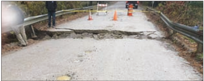
The bridge on Red Fox Crossing in Hillsborough is out. Residents must detour to Hummingbird Lane to get around.
