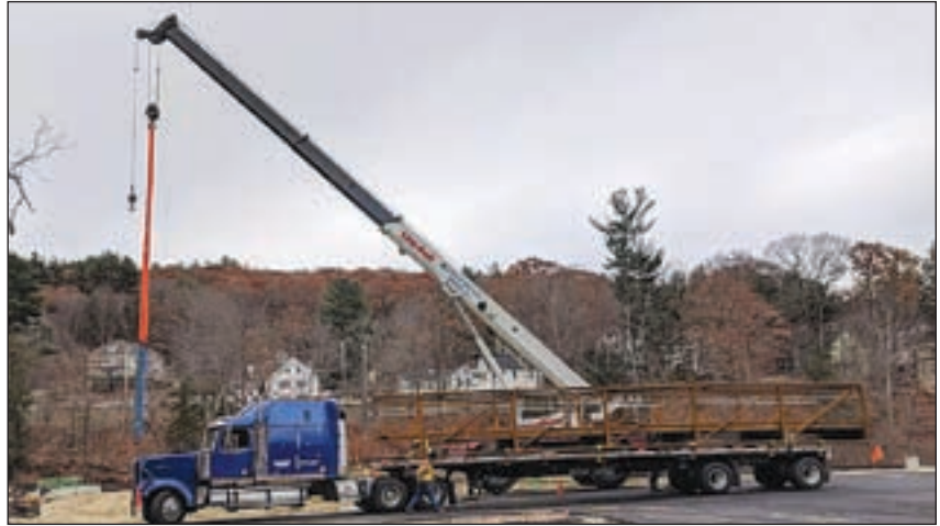
Segments of the new footbridge, which will connect Depot Square Park with the new Riverwalk parking lot have arrived and are in the process of being unloaded & joined, and are scheduled to be installed this week. (weather permitting).
