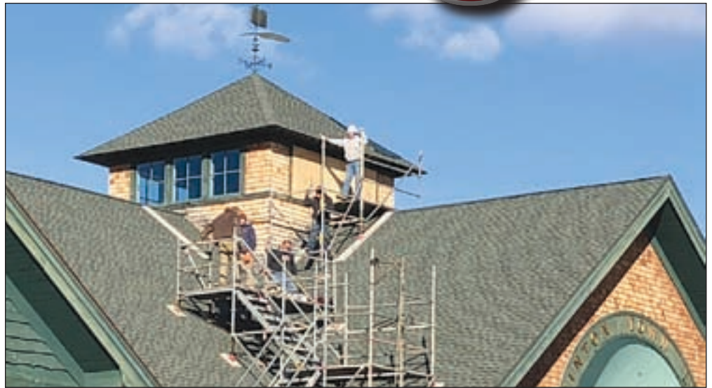
Progress continues on repairing the fire damage to the Hopkinton Library as crews begin replacing the roof on the cupola.
