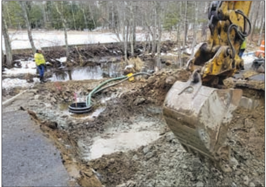
Goffstown's DPW installed a new concrete box culvert on Stinson Road right at the beaver dam over the last few weeks. This new 3' x 6' box culvert replaced two failing 18" pipes. Next year guardrail and top coat of pavement will be installed.
