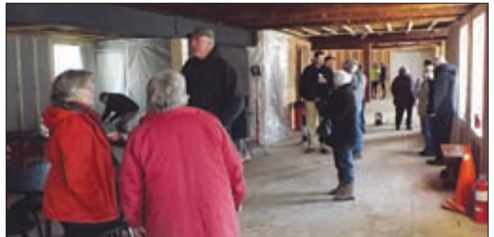
Progress at renovating Francestown's Village Store was evident at Saturday's Open House.
