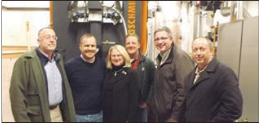
John Stark High School held an Open House to celebrate the completion of its new Biomass Boiler. Those attending included Stephen Eckberg, Public Utilities Commission; Zack Lawson, School Board Chair; Superintendent Dr. Lorraine Tacconi-Moore; John Astholz, Stark Facilities Director; Michael Davey, EEI, Inc; and Mark Froling, Froling Energy.
