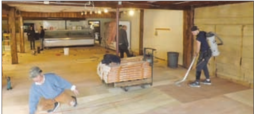
Renovations at Hopkinton's Cracker Barrel continue at a feverish pace to meet the April 15th soft reopening.
