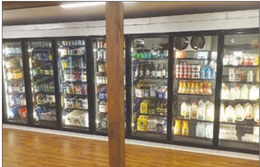
With the installation of the coolers, renovations at the Cracker Barrel are nearly complete and the store is open for business.
