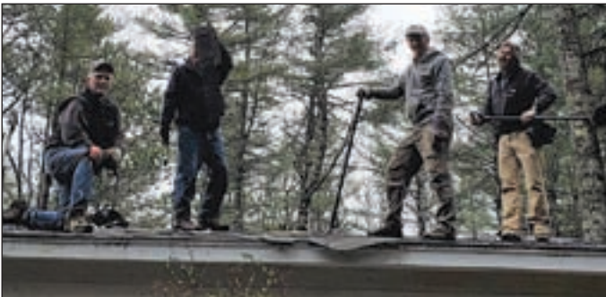
Hopkinton Rotary Club's roofing crew helped out a senior citizen in need.
