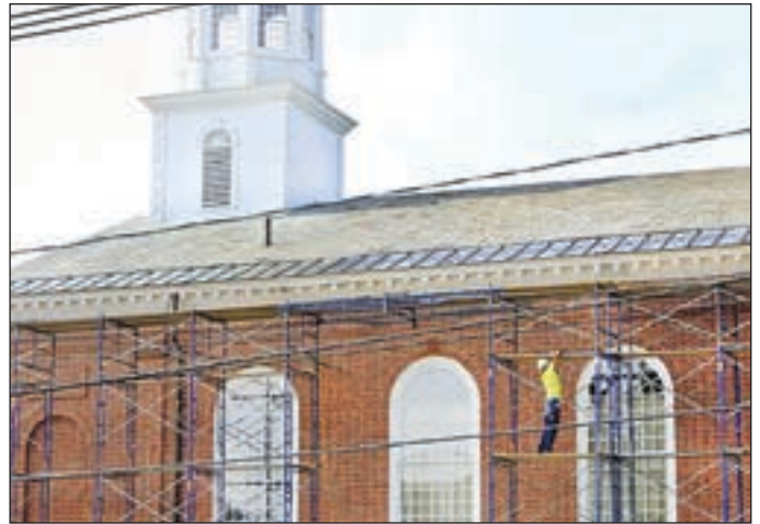
Crews are replacing the 100 year old slate roof on the south side of the Peterborough Town House. Work on the north side will be completed soon.
