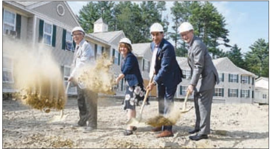
Summercrest board member Vern Violette, CFO Jean Shaw, board member Dan Hassan and CEO Steve Gunnerson shovel dirt at the Summercrest groundbreaking in Newport August 8. Summercrest is adding on an addition and renovating the existing building to add 28 more beds, add a new all day cafe market, expand the recreation area and add a raised patio to the assisted living facility. The work is anticipated to take about a year to complete. Paul Howe photo.
