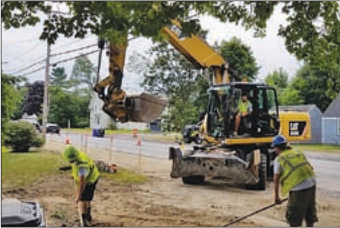
Last week Goffstown DPW paved sidewalks and driveways on the outbound side and constructed wingwalls around new drain pipes on the box culvert near Summer Street. Remaining yards were all loamed, hydroseeded and staked/ribboned off. The focus is North Mast and overlays on major roads before school starts.
