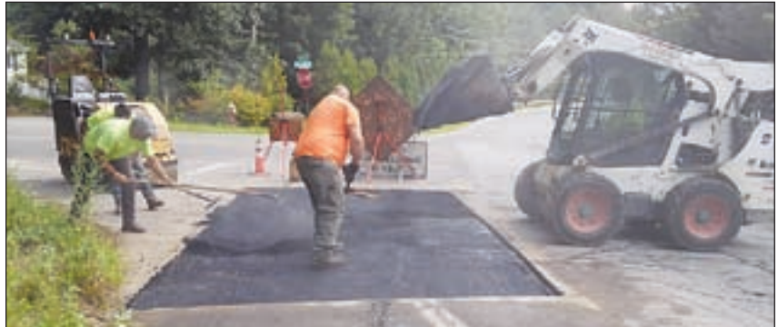
Goffstown DPW completed permanent trench patch paving on Elm Street last week along with final cleanup and punch list items. Public water is active, tested and being used at the DPW facility and has also been extended to the proposed sports fields for future irrigation use. This project is now complete.
