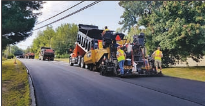
Goffstown GPW has installed a shim layer on Daniel Plummer before the final top course overlay.
