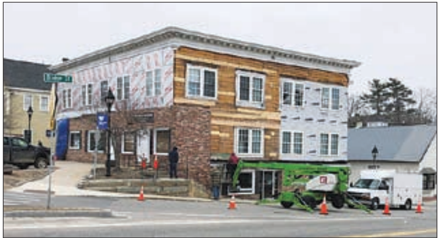
In addition to back-side repairs after a recent fire, a Henniker landmark is getting a major facelift.
