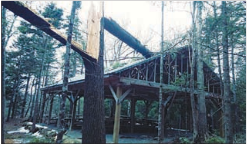
Washington's historic Seventh-day Adventist Church site was closed to visitors while workers were there to remove the tree that fell on the pavilion and repair it.
