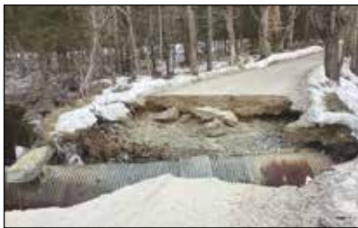
Heavy rains caused this washout on Hillsborough’s Stowe Mountain Road.
