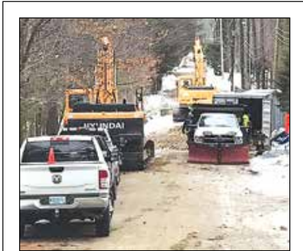
Work has begun on the Red Fox Crossing Bridge at Emerald Lake with completion in March.
