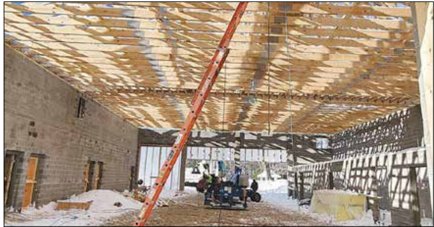
The rafters have been installed on the truck bay of Newbury's new Fire Station.
