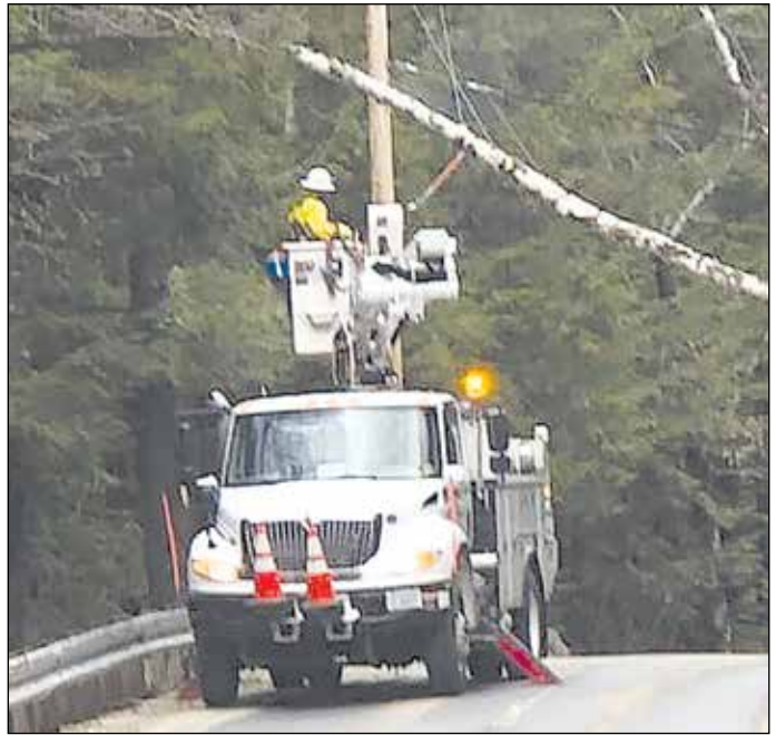
Newbury Fire Rescue responded to a call for a tree down blocking the road with wires down on Monday evening. Responders found a large tree completely blocking Morse Hill Road with wires down. The road was blocked and Eversource was notified. The utility responded within the hour to remove the tree and restore power. If you see a tree down with wires, please stay clear and call 911. Always assume that the wires are live.
