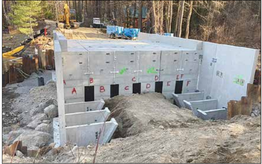
Progress is being made on the Red Fox Crossing Bridge at Emerald Lake.
