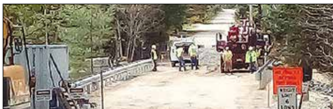
Plans call for the Red Fox Crossing Bridge at Emerald Lake to reopen Friday the 14th.
