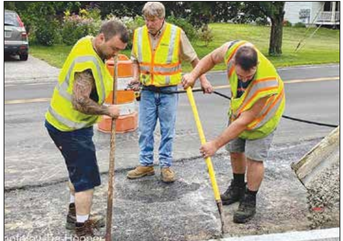
Hats off to Leo Aucoin and his Henniker Highway crew who worked Saturday in oppressive heat to complete the curbing installation, which needed to happen to prepare for the sidewalks and get ready for the final topcoat on Monday and Tuesday. They are true Public Servants.
