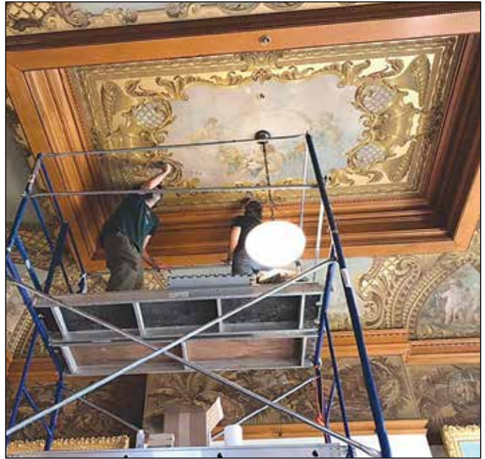
Conservators Wenda and Gregg are back cleaning and repairing the painted ceilings and woodwork in Fuller Library's Bio Room. Special thanks to the NH Council on the Arts for the Mooseplate Grant and to the Town of Hillsborough.
