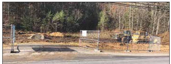
Ground has been broken for the new Aubuchon Hardware Store on Route 114 in Weare.
