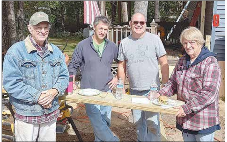
The Concord Region Habitat for Humanity has been rehabilitating a home in Warner for a family in need. Here, L-R, volunteers Don Lassonde, Eric Weiner, Mark Tierney and Barbara Lassonde take a break from building a wheelchair ramp.
