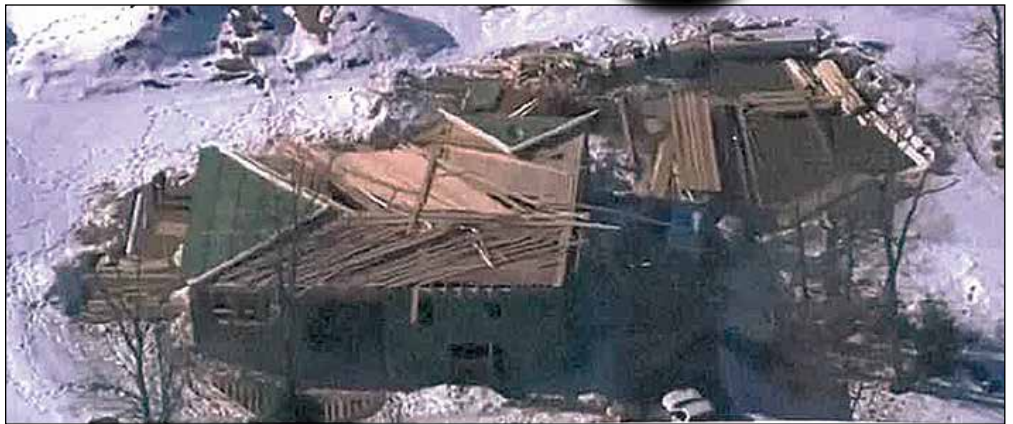
Two construction workers were injured when this Bennington roof collapsed.
