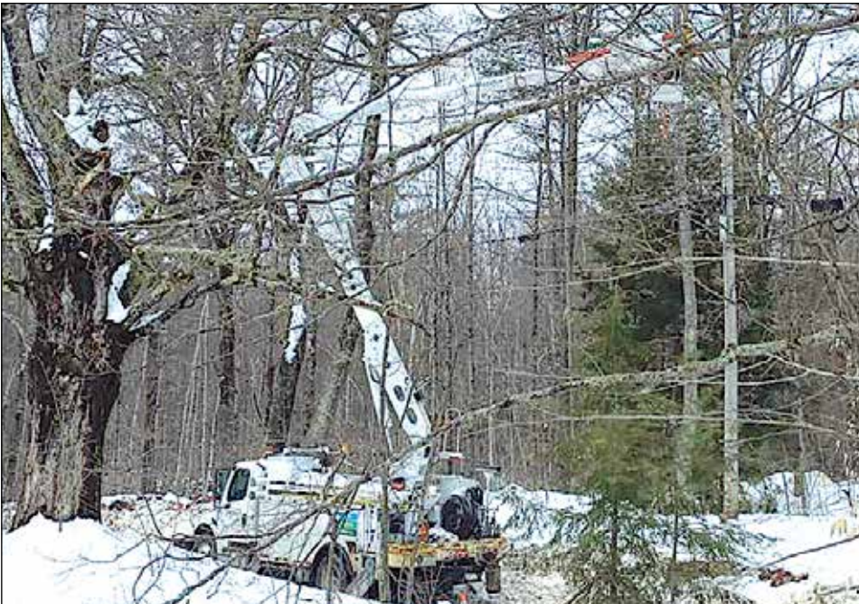
Eversource brought in utility crews from across the county to deal with downed trees blocking roads and disrupting power.
