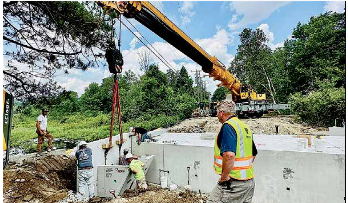
Henniker’s Highway Crew is working on the Liberty Hill Project. The Precast Bridge, made by Michie Concrete Products, was installed by teams from Hall’s Excavation and Michie Concrete Products.
