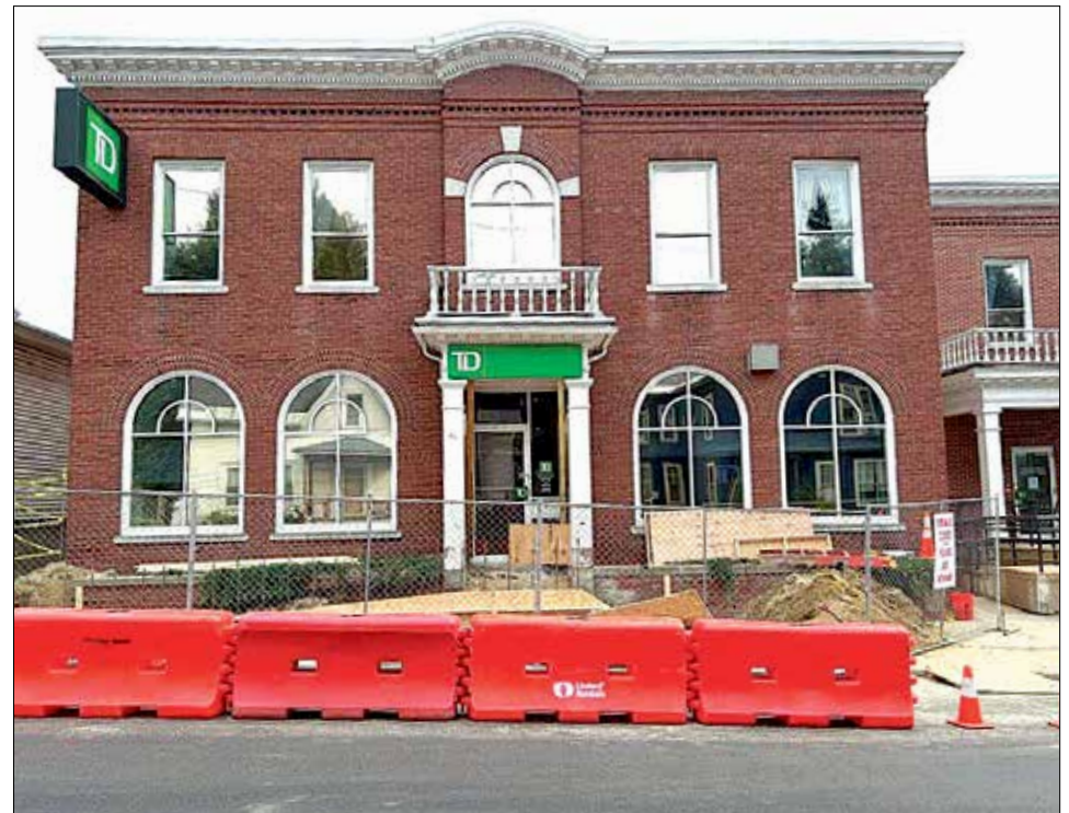
The main entrance to Hillsborough’s TD Bank is closed as the sidewalk and stairs are being reconstructed. Patrons are urged to use the side or rear entrances.
