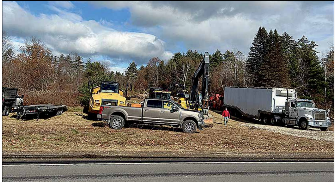
Avanru Development Group, Ltd. has broken ground on its Hillsborough Heights Phase I project of forty-two state of the art, energy efficient workforce housing units expected to come online in 11 months.
