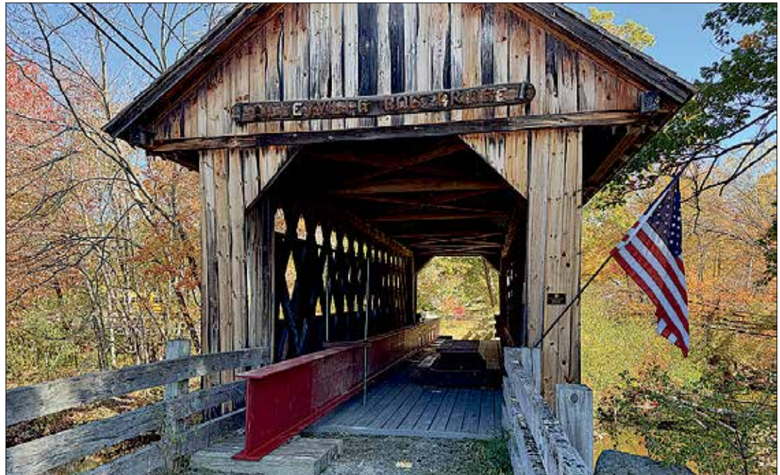
The Andover Select Board was informed that the Hall Street Bridge membrane was installed and the paving was completed. Also, the Cilleyville Bridge (shown above) steel beam was placed to help save the bridge for the time being.
